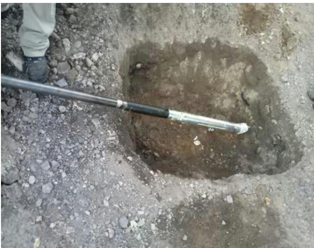
For difficult underground – backfilled ground and gravelly ground – a 3-fingerhead was used, which drills this underground without any trouble.
