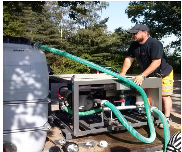
The mixing + pumping station can easily be operated from the loading platform of the truck.
