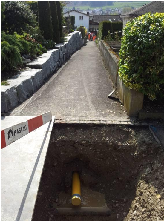
The pulled in HDPE pipe in the arrival pit. The complete 49 m (160 ft) long bore including pipe pulling took half a day.
