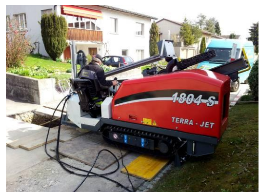
Here drills the boss! Christian Salzmann drills concentrated during the pilot bore.
