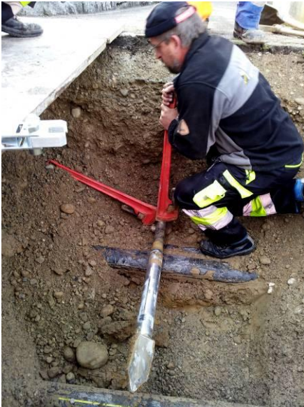
The drill head reaches the arrival pit right on target. The backreamer \varnothing 160 mm (6.3") and the HDPE pipe \varnothing 125 mm (5") are assembled and pulled in.
